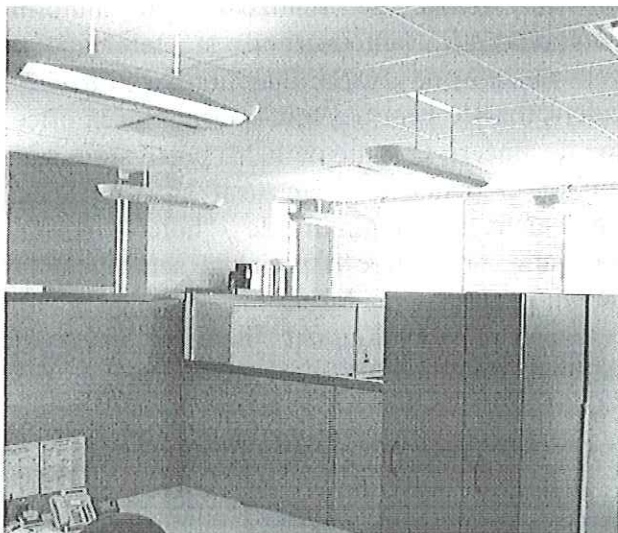
Figure 2 Ergolite's occupancy sensors save energy by turning off desktop lights over vacant spaces
